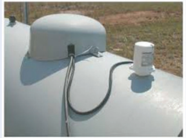
Tank monitor on top of LP tank
